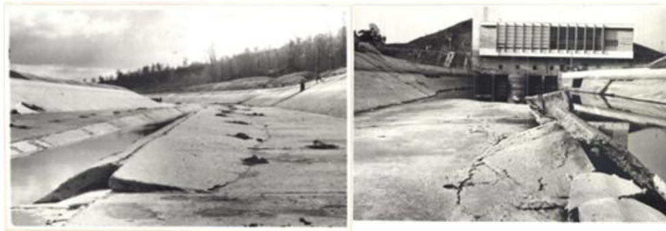
Fig. 2. Severe damages of tailrace channel.
