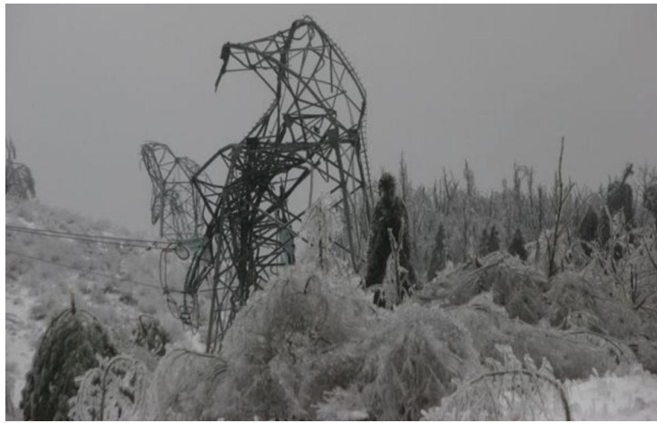
Fig. 6. Icing of an overhead line.
