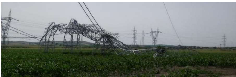
Fig. 5. Breakdown of an overhead line due to a tornado.
