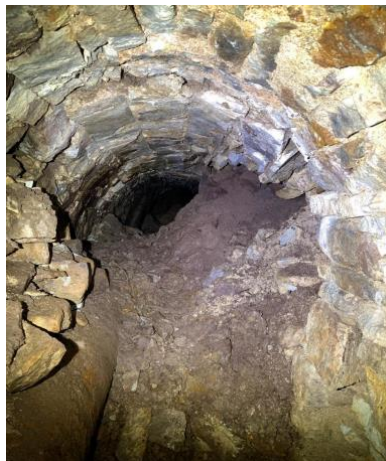
Fig. 6. Local failure of bottom outlet gallery.
