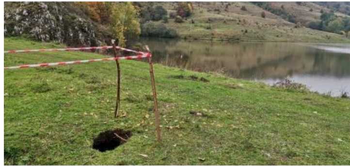
Fig. 5. Sinkhole at dam's crest during Taul Mare Dam incident (Oct. 2022).
