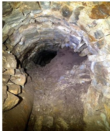
Fig. 6. Local failure of bottom outlet gallery.
