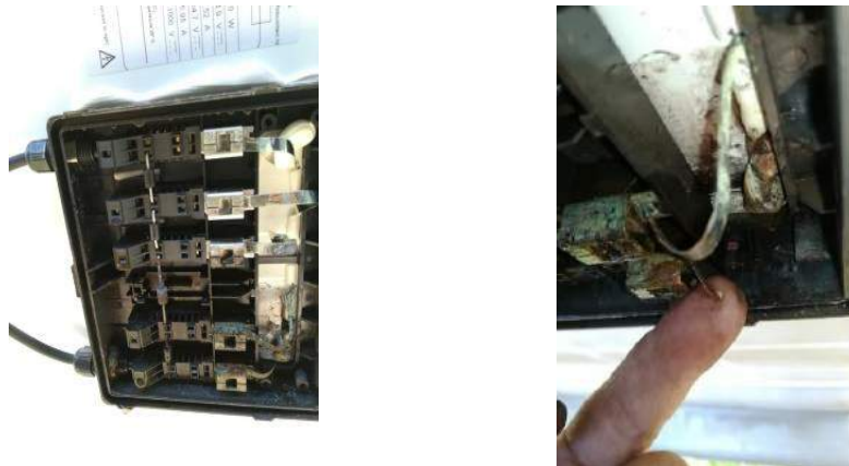
Fig. 20. Damaged junction box by water penetration.
