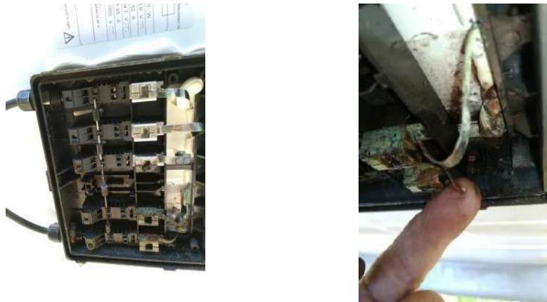
Fig. 20. Damaged junction box by water penetration.
