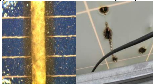
Fig. 17. Degradation of cell connections produces an electric arc or hotspot that causes burning of the back sheet and interrupting the modules string.
